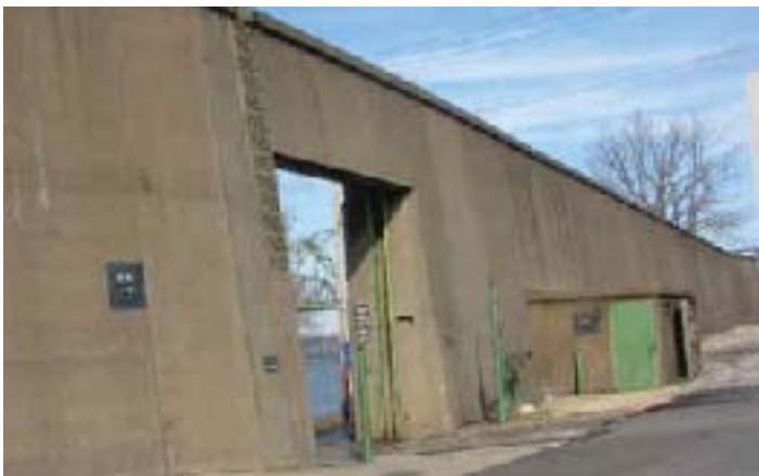
Fig.6_9 : permanent floodwall @ parkersburg, WV
